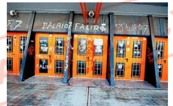
Graffiti covers a stadium at the Faliron site Image source: http://www.dailymail.co.uk/news/article-1036373/Abandoned-derelect-covered-graffiti-rubbish-What-left-Athens-9billion-Olympic-glory.html#ixzz1jT6eXAh
